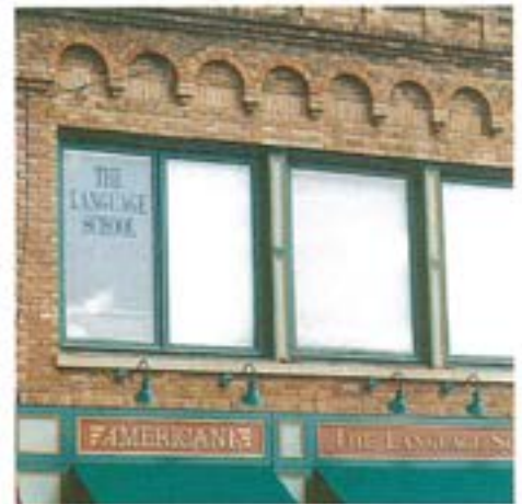
Some punched windows can include very flat arches but not round ones.
